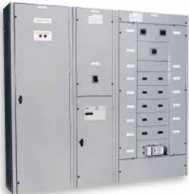
Fig. 16 Transfer switch with distribution.
