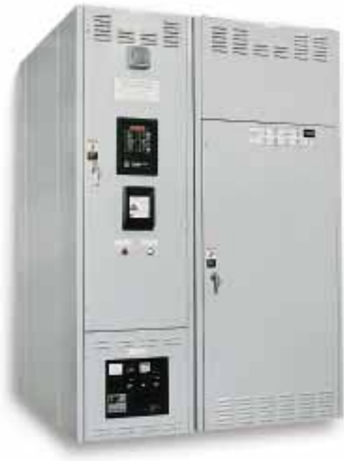
Fig. 7 Two source system with main circuit breaker, protective relaying and automatic transfer switch rated 1200 amperes.
